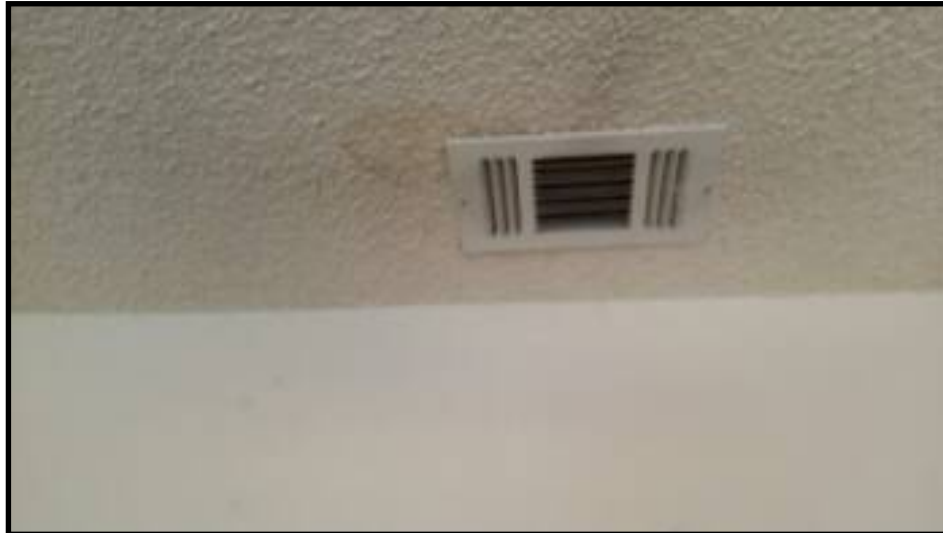
Small stains noted on the ceiling. They tested dry at the time of the inspection.
