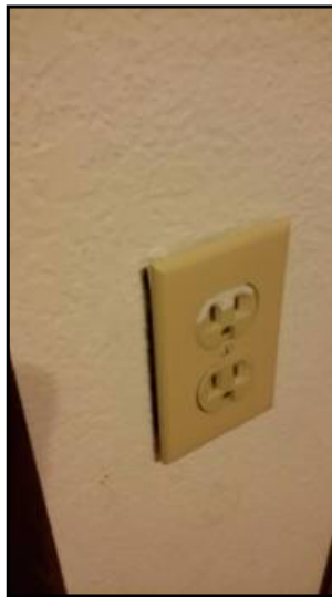
Loose outlets noted.
