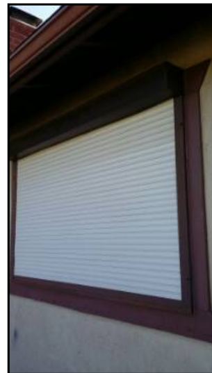
Window hardware damaged.
