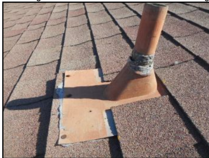
Exposed nails on roofing material. Recommend sealing all fastener heads.
