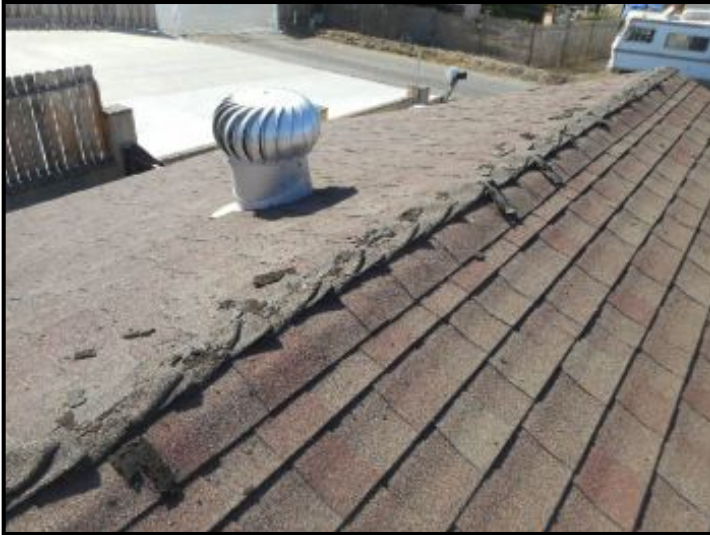
Some shingles damaged.
