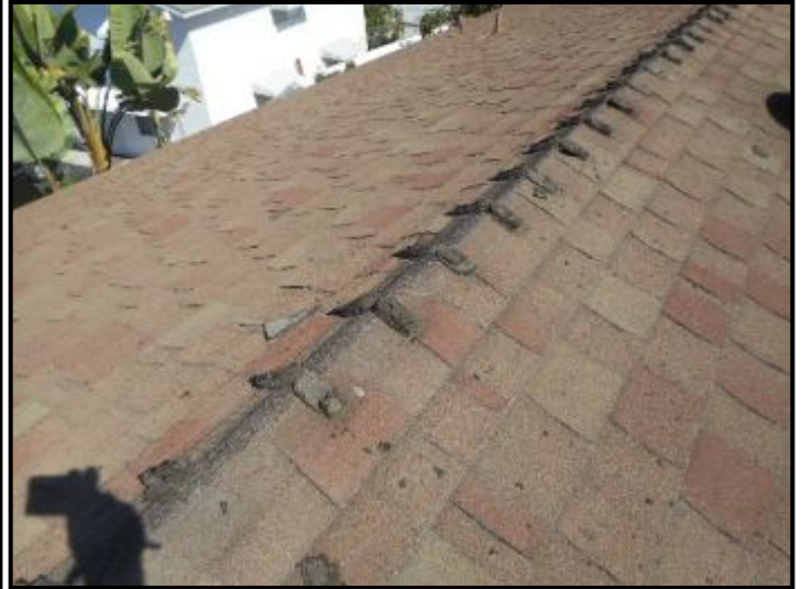
Some shingles damaged.
