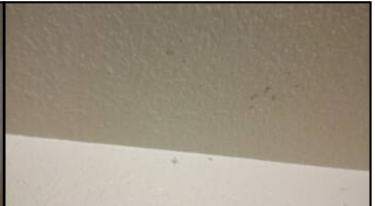
Mold like stains present on the ceiling. We recommend having a mold sample taken and lab tested, also monitor the area for water intrusion.
