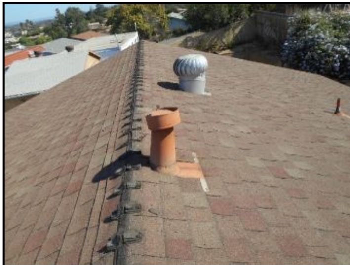
There are loose B vent caps noted. We recommend refastening the vent caps.
