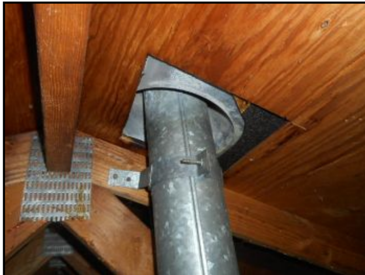
Evidence of past or present leaks, dry at time of the inspection. Monitor for leaks &/or have roofing contractor evaluate.
