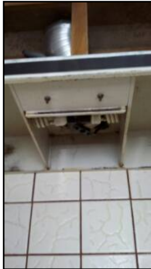
Exhaust fan is inoperable.
