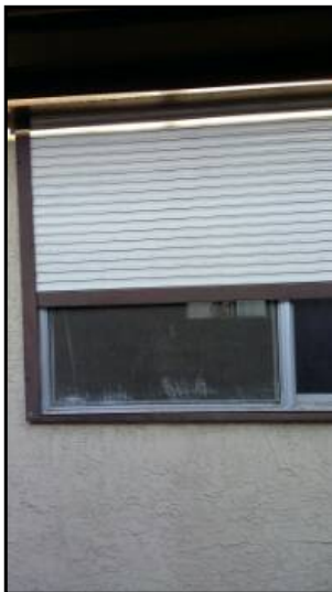
Some window screens damaged.
